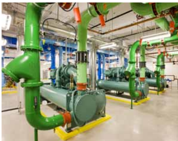
A chilled water cooling system more efficiently supports HPC environments
